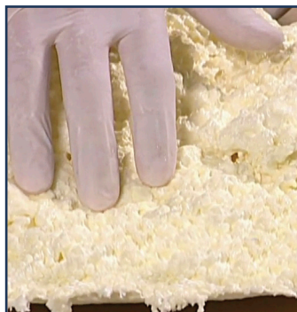
Off-Ratio, more "B" chemical is being dispensed
